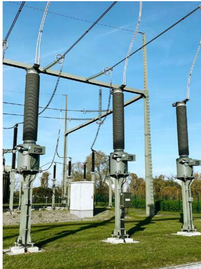
FIG. 27 Voltage transformers with climate-neutral insulating gas synthetic air at Amprion
