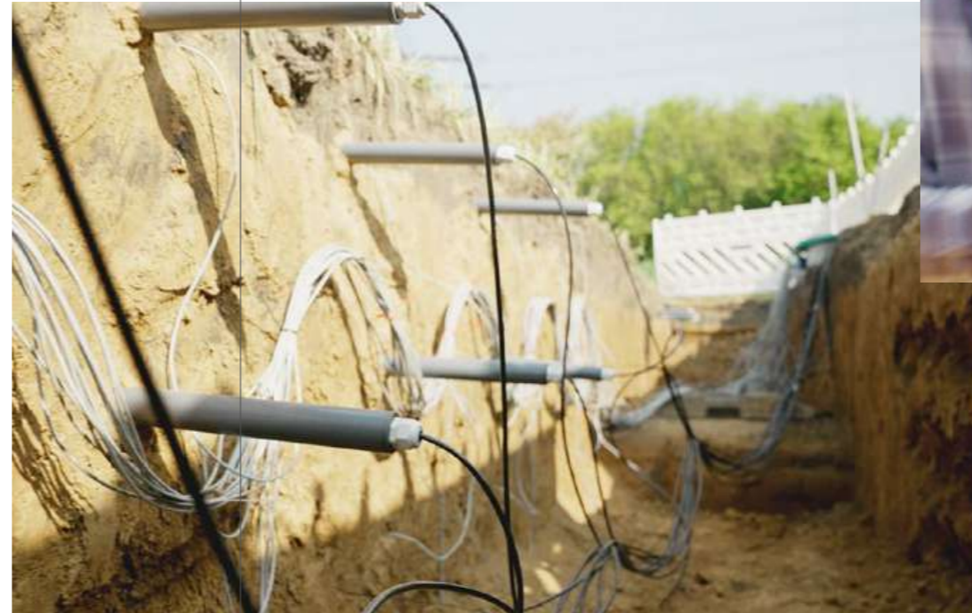
FIG. 35 LEFT Measurement probes for monitoring soil moisture and temperature FIG. 36 TOP Installation of measurement probes in the control area
