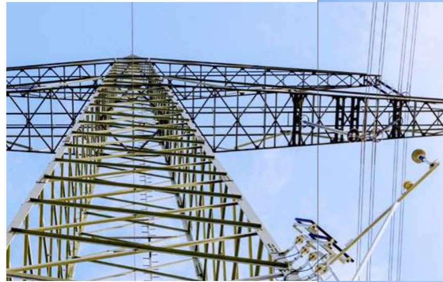
FIG. 33 AND 34 Amprion weather station on an electricity pylon
