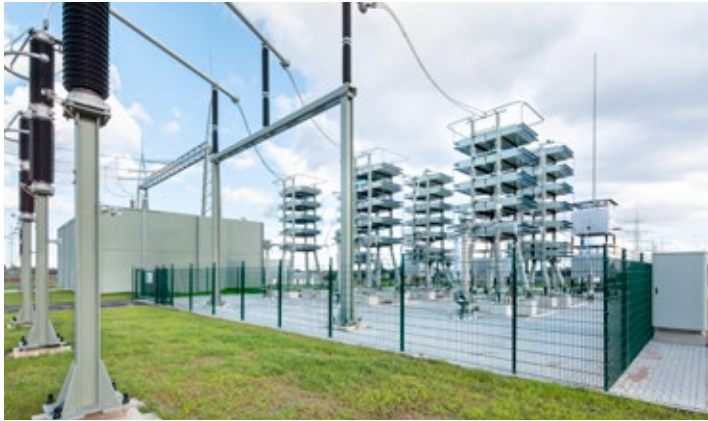
The most powerful hybrid substation in the European power grid is located in Kriftel. From here, Amprion stabilises and secures the power supply for the Rhine-Main region.
