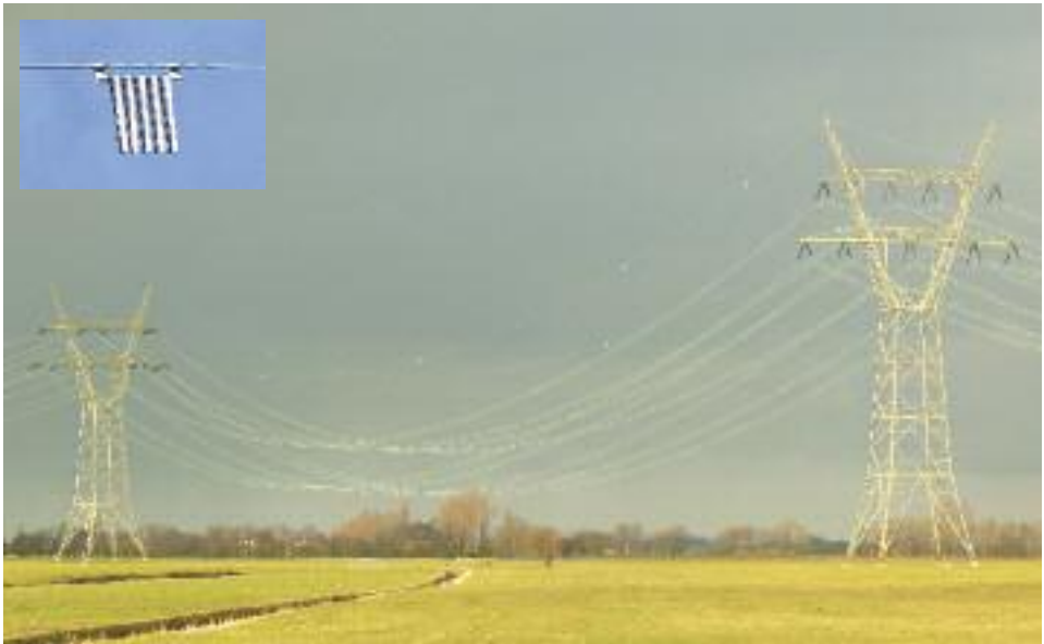
Figure 4: High-voltage (150 kV) power line in the Netherlands, with bird flappers (see inset) placed at regular intervals along both ground wires as bird flight diverters.
